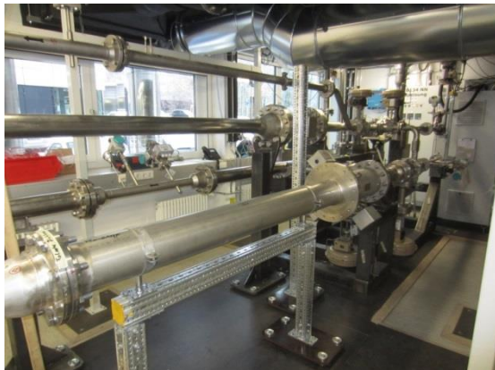
Figure 4: Set-up of the MGT test rig (without insulation)
