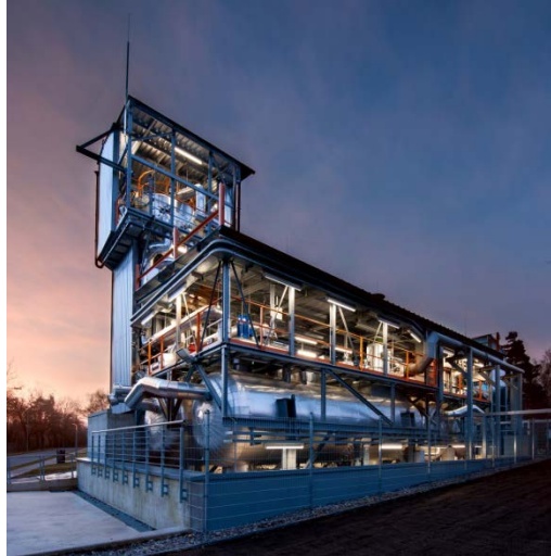
Fig. 1. TESIS:store test facility with thermocline storage tank (inside the tower) and cold and hot reservoir tanks in front
