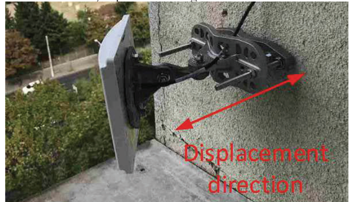
Fig. 5. Displacement direction of TX1 antenna
