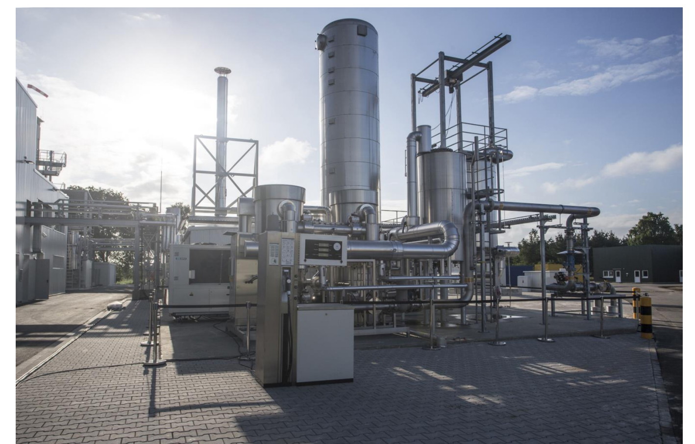
Fig. 4: Photo of existing Audi e-gas plant in Werlte, Germany
