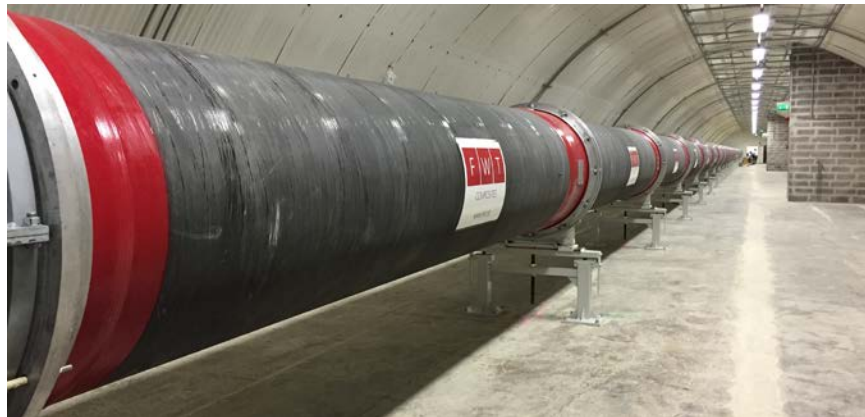
Figure 1: Photograph of the 115 m long CICLoPE facility with the measurement location seen at the far end
