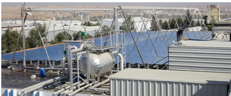
Fig. 1: Collector Field and Steam Drum on the RAM Pharma Rooftop
