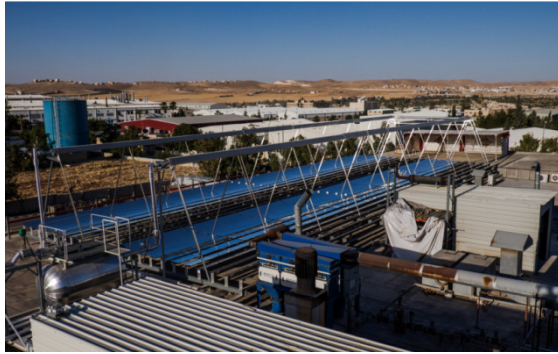
Figure 2: Fresnel collector at RAM Pharma
