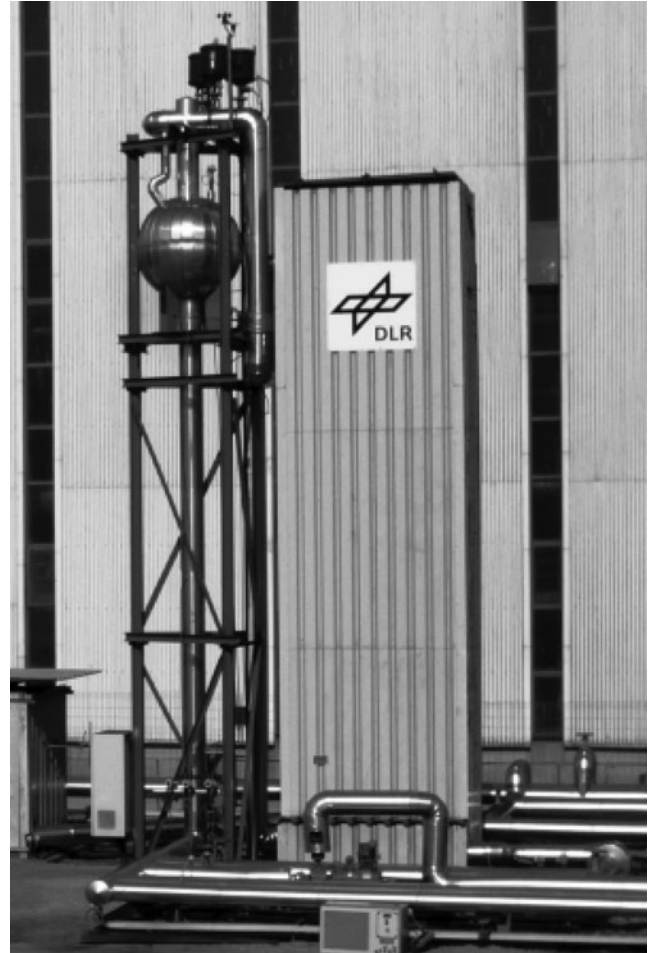
Figure 3 PCM storage in the water/steam test loop at the Litoral power plant of Endesa in Carboneras, Spain.
