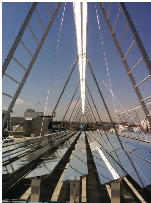
FIGURE 3. Image of one of the two collector strings in operation. Picture taken, when first solar generated steam was delivered to RAM Pharmaceuticals on March 17 th , 2015.
